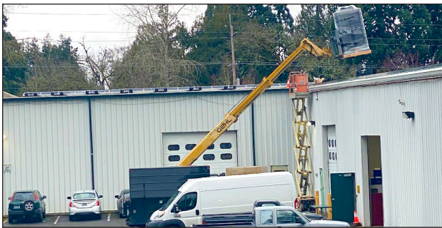
Several solar panels were installed on the roof of Shangxi-La's Salem Administrative Office in March.
