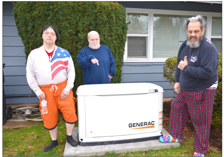
(Left to right) Tom, Steve P, and Steve M stand next to the GENERAC standby generator installed at their home in south Salem. The generator is one of eight generators installed at Shangri-La residential programs.
